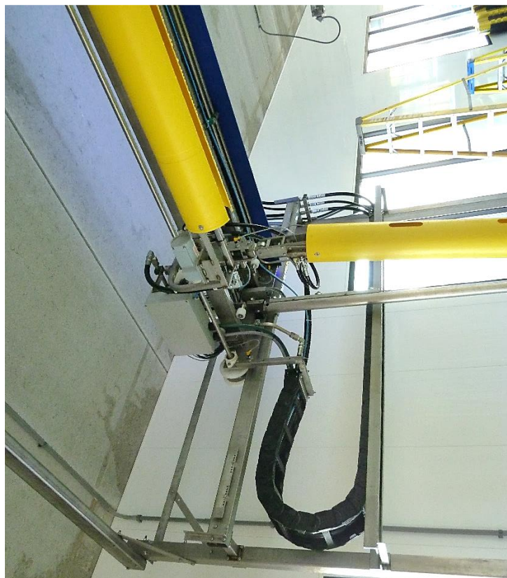
Main Rail, P.S. Exit
